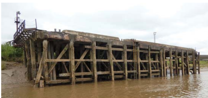
Gunness Wharf Fina Oil Jetty
